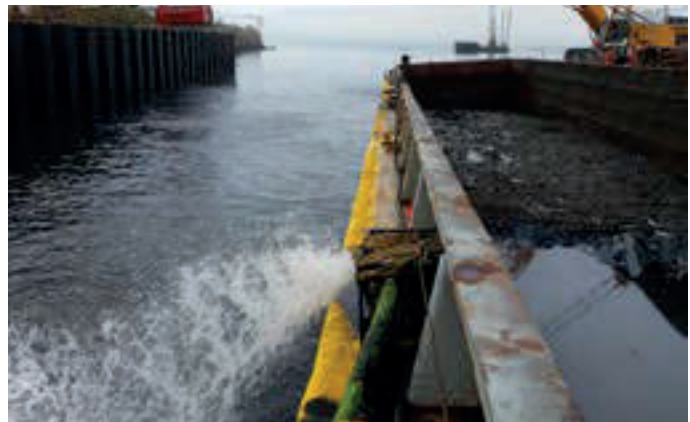
Clean water discharge decanted after treatment
